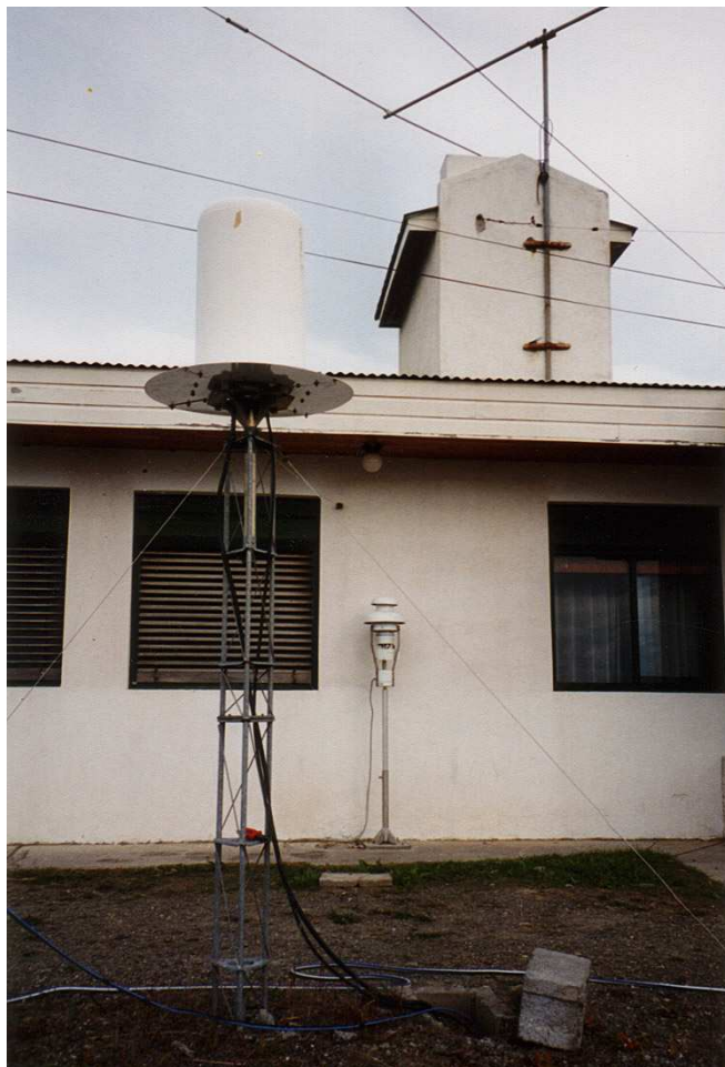
Initial installation (1987): Alcatel antenna, very loose guying
