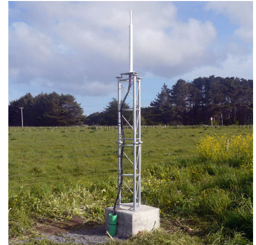
Type III (29%): very rigid steel tower on concrete block
