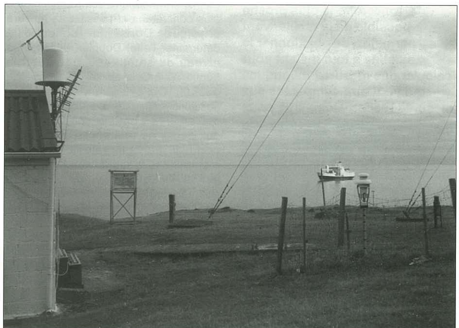
The Doris beacon attached to the island radio shack at Tristan da Cunha. On the right is the Doris met package surrounded by wire to keep out cattle. Next to the wall can be seen the 17 batteries supplied by IGN to power Doris over-night; these will also be protected from cows and the weather. The second antenna on the roof transmits tide gauge and met data to POL via Meteosat. In the background can be seen the RMS St.Helena.
