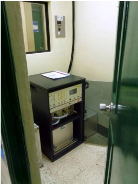
The DORIS beacon at INETER headquarters
